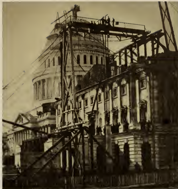
A marble monolithic column for the Senate portico is swung into place. In the background the dome nears completion.
